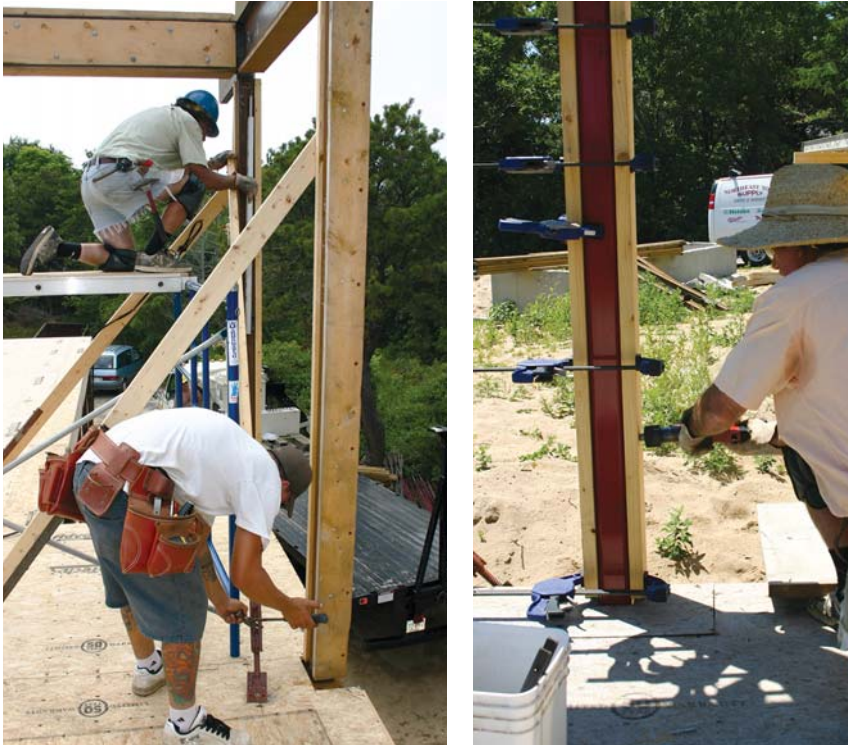
Figure 7. Adjustable form braces provide the fine-tuning required to compensate for the jostling that occurs when heavy perimeter beams are set (left). The author clamps 2x6 cladding to a column and secures it with powder-actuated pins (right).
