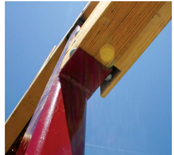
Figure 6. Where an LVL header meets the steel post, the author welded 3-inch-deep bearing plates to support the beam. Though the LVL adds no structural strength to the frame, it matches the column thickness and provides stiff backing for the finish trim.
