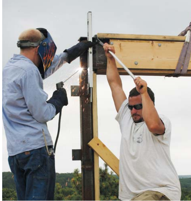
Figure 9. Because steel parts tend to pull toward the bead during welding, a worker uses an extension handle on the rigger's wrench to steady a beam while the welder applies a tack.
