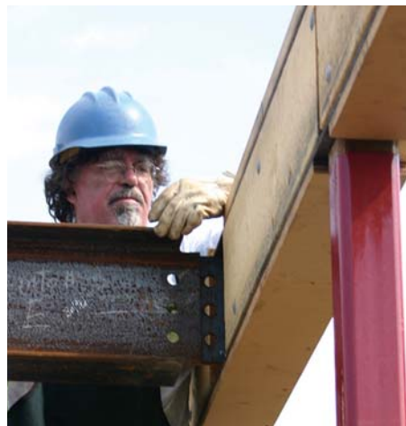
Figure 4. Bolt-on angle clips can support wood framing, as in the case of this LVL stairwell header (far left). A welded bolt flange (left) stiffens the beam web beneath a second-floor column location and also supports a right-angle beam.
