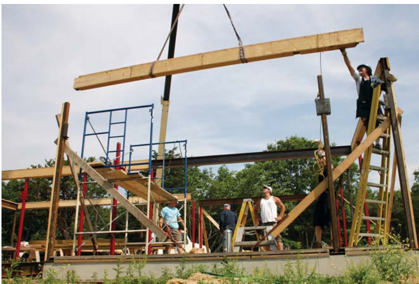
Figure 8. Working with a 68-foot boom, the crew set the first-floor perimeter beams in one long day. Installing the wood cladding while the steel was still at the shop saved plenty of on-site labor.
